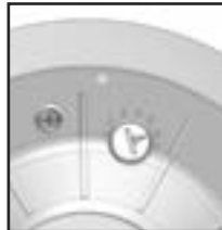
Transformer adjustment from front.
